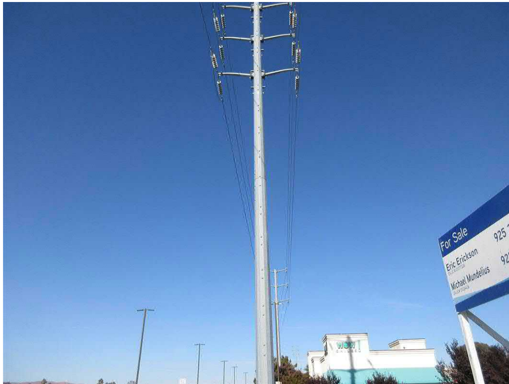
Photo 9: View of the utility pole and electrical transmission lines located in the southwestern portion of the subject site.
